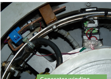
Generator winding exciter
