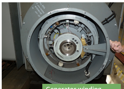
Generator winding exciter
